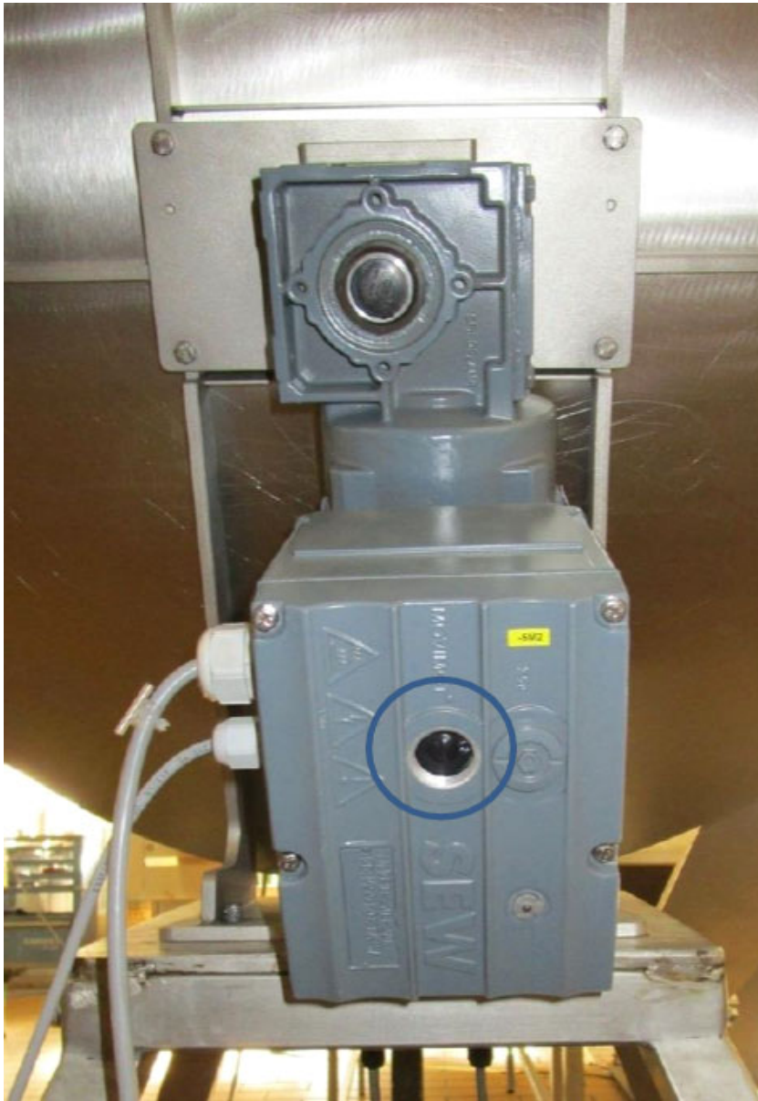
Figure 8-2: Hopper Drive, Frequency Inverter with Cover unscrewed
